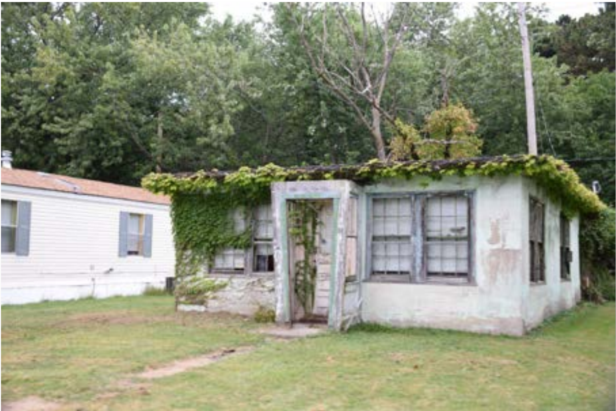
Concrete Cottage, early 20 th Century and its present condition
